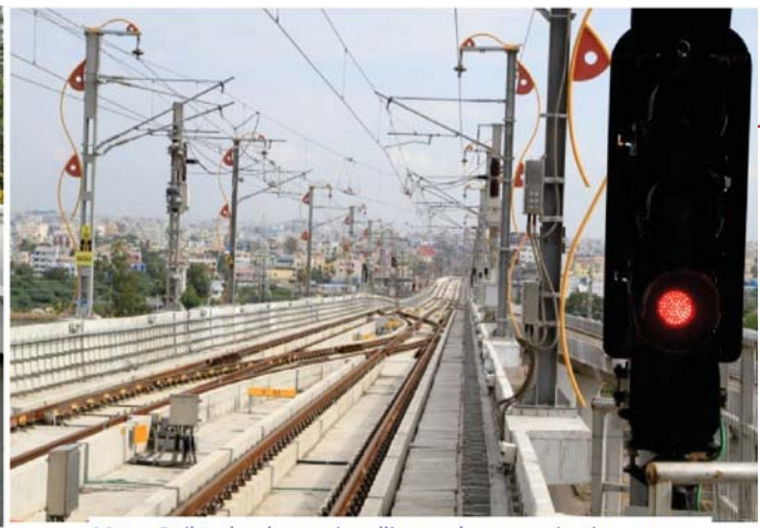
Metro Rail technology –signalling and communication system
