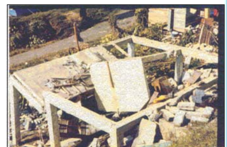
Pictures showing the effect of cyclone on structures
